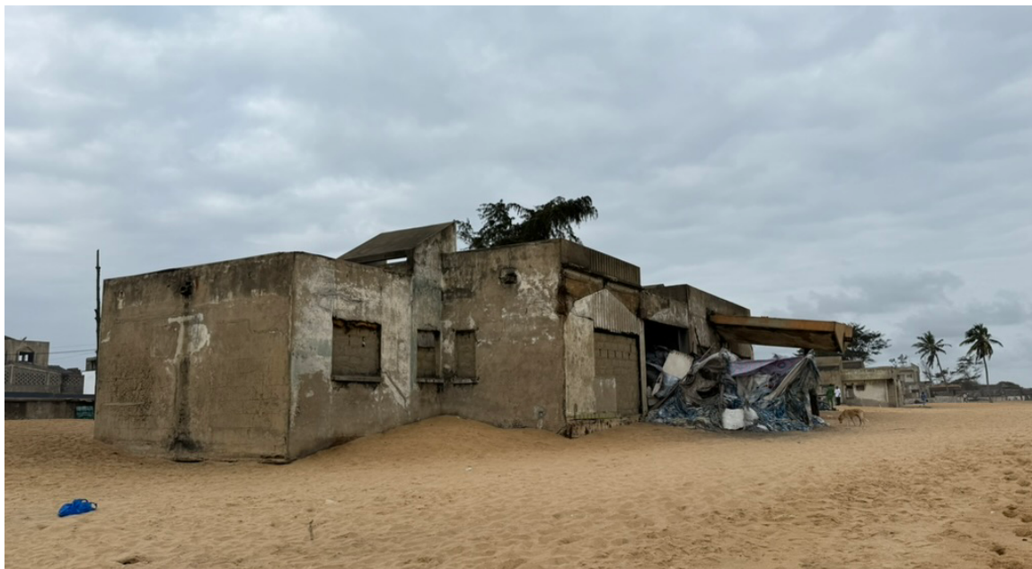
Erosion-damaged infrastructure on the Benin coast a stark reminder of the climate adaptation imperative facing African communities.
